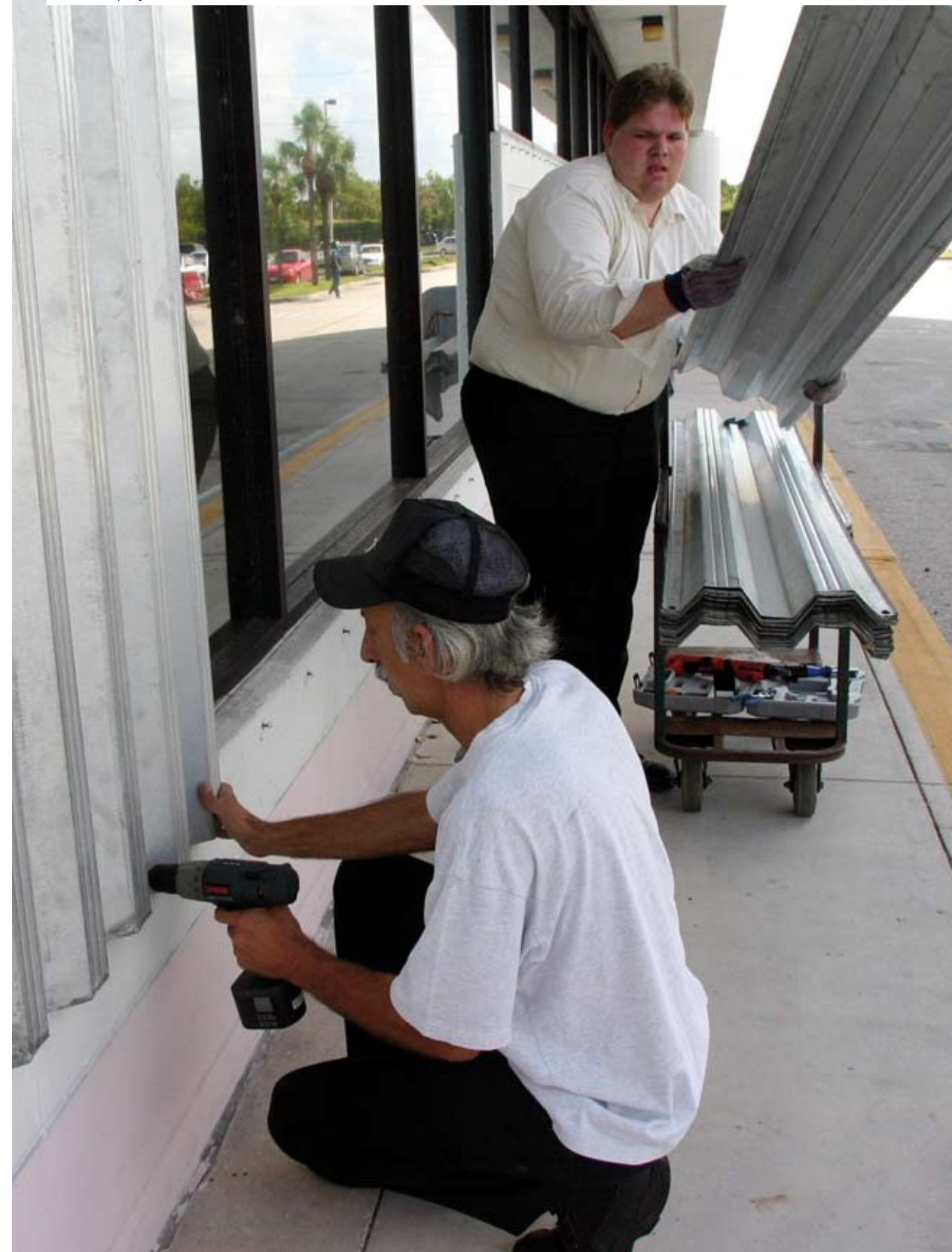
Store employees install shutters for Hurricane Jeanne in Florida, USA. Photo: Reuters/Marc Serota
