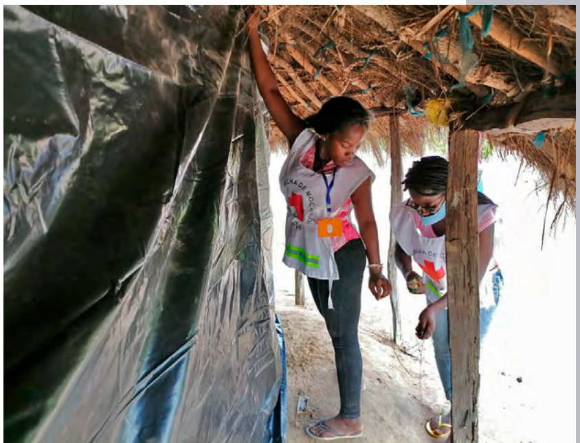
The Mozambique Red Cross strengthened shelters for 1,500 families in December under the IFRC's DREF forecast-based action protocol as Cyclone Chalane loomed. (IFRC)
